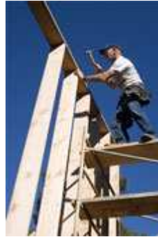
PPE and Fall Protection missing
