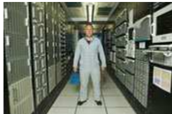
Clean computer rack areas
