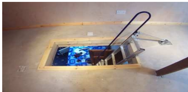
Non Compliant Floor Opening
