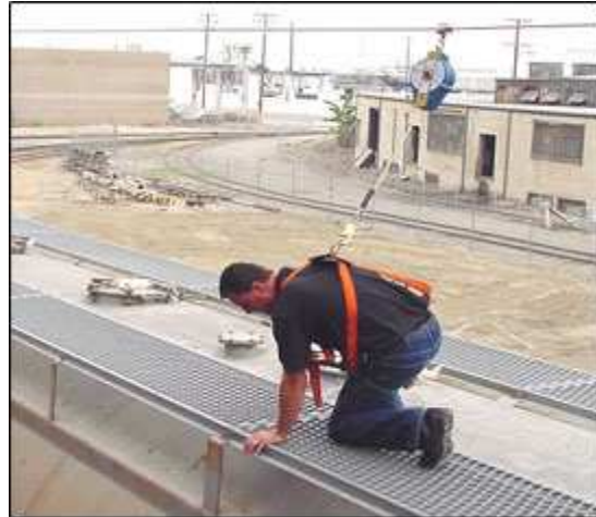
Secured to Fall Arrest System Hard Hat missing MUST be worn
